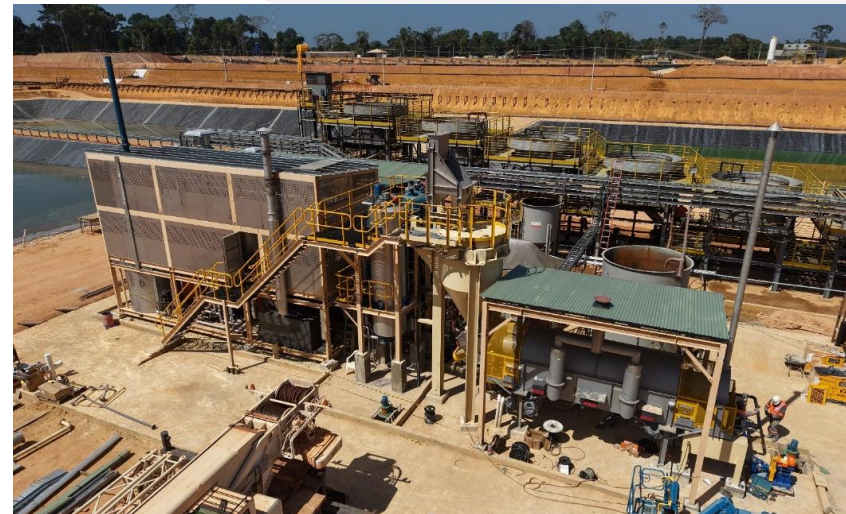
ADR and CIL columns in wet circuit area
