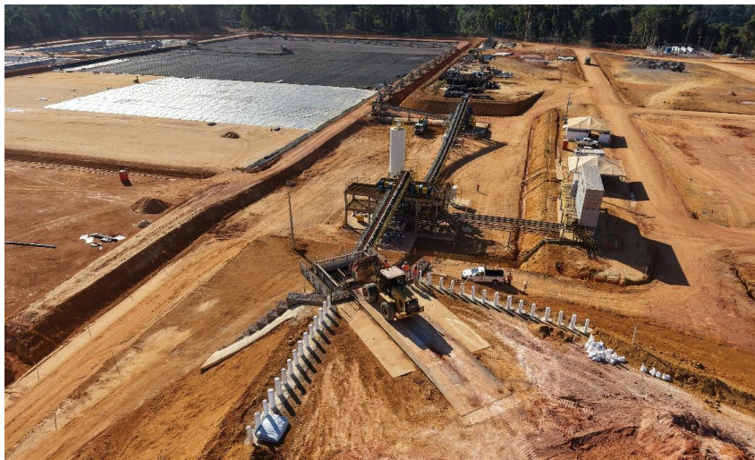
Dry circuit showing ROM ore bin in foreground, sizer and cement silo and agglomerating drum and conveyors
