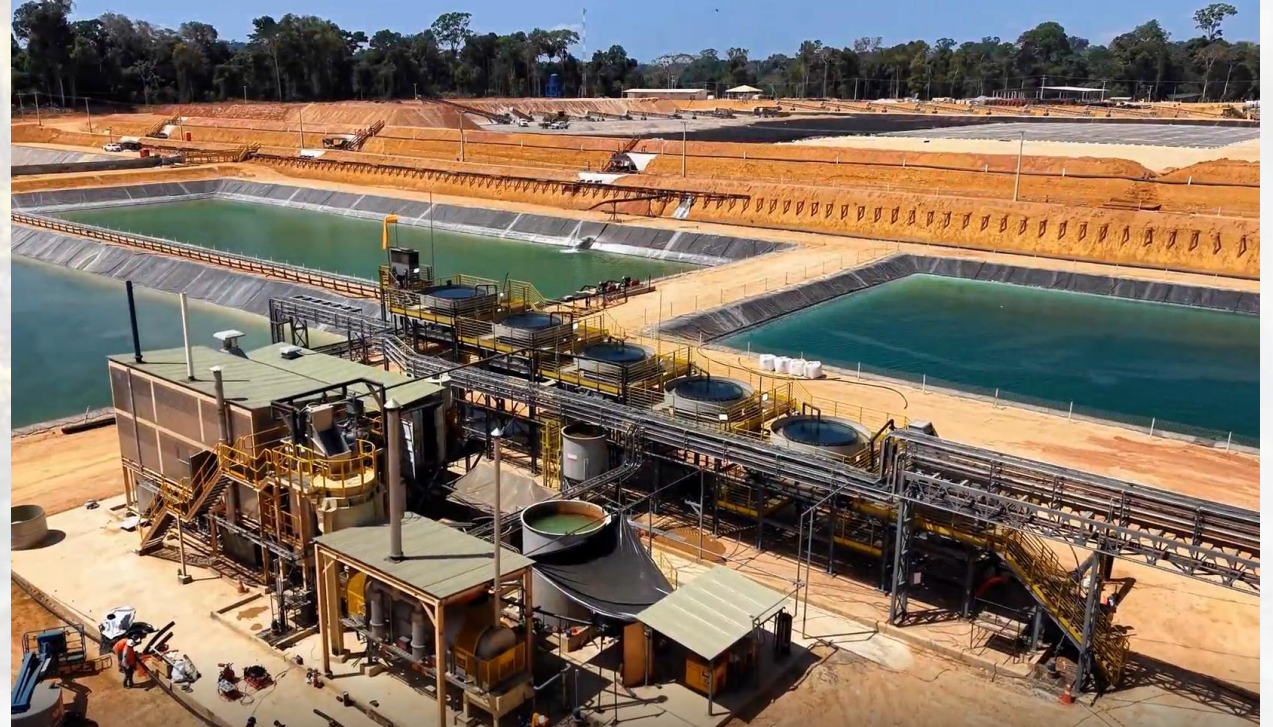
ADR and CIL columns in wet circuit area together with solution ponds and heap leach pads in background
