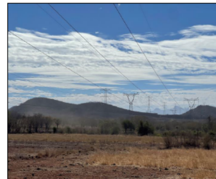
High voltage national grid near site
