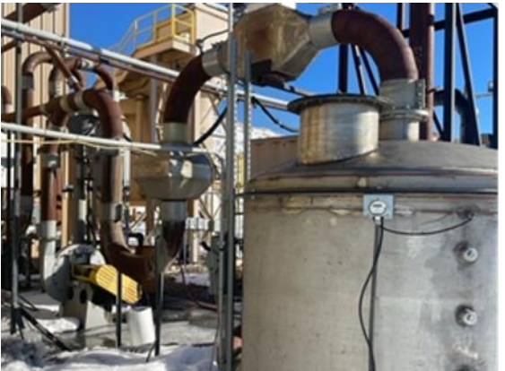
Deep Bed Scrubber
