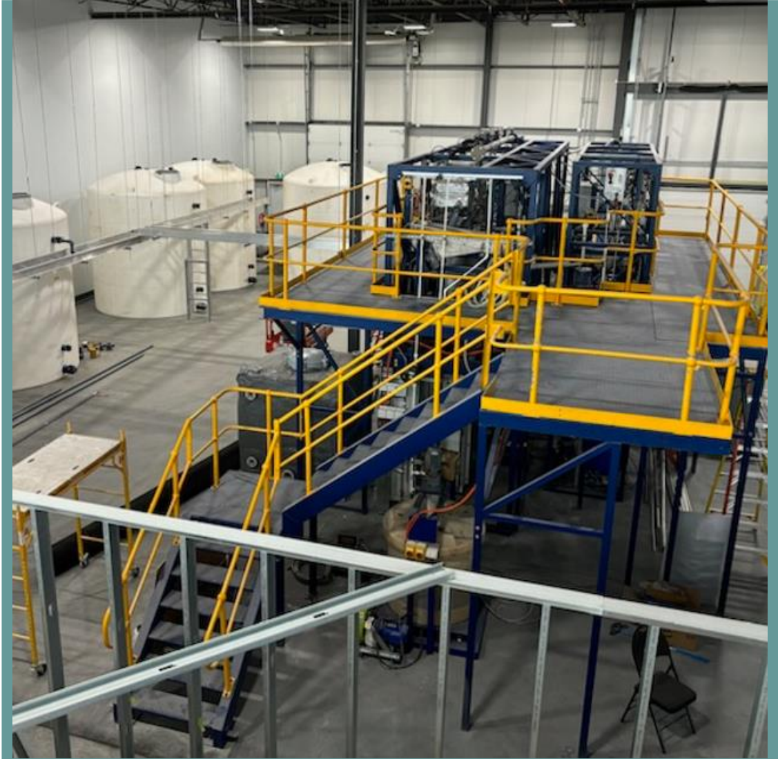
LithiumBank received its Pilot Plant in January 2024 and is in the process of installation & commissioning. Photo dated March 28, 2024
