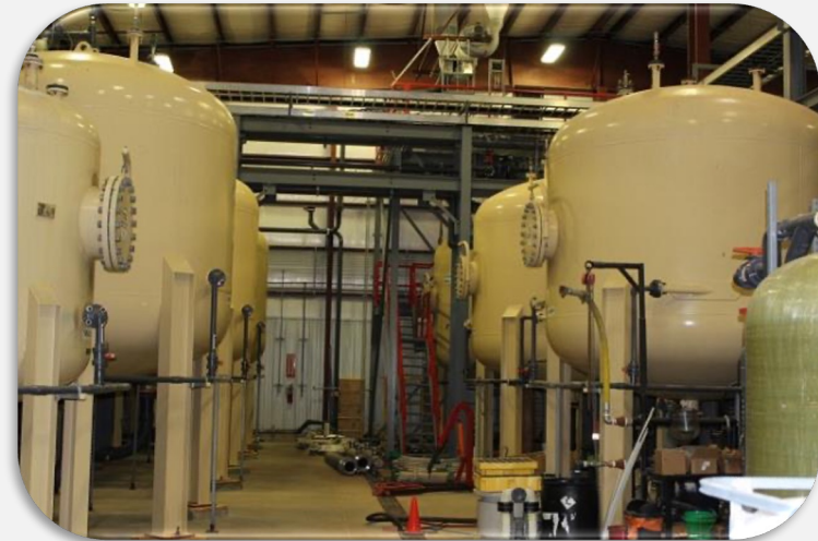
Lance Satellite Plant Ion Exchange System
