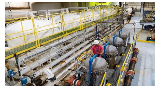
Christensen Satellite Plant Interior
