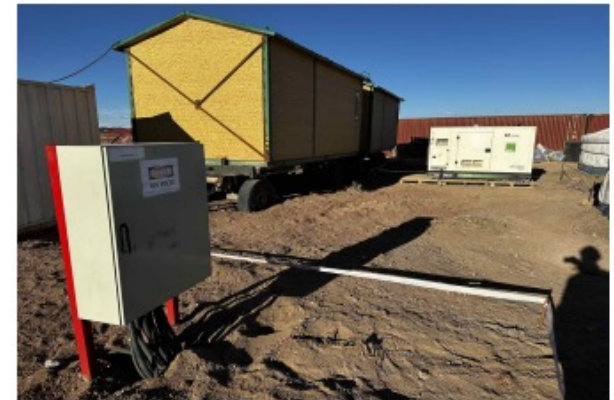
Ger Camp & Construction Power
