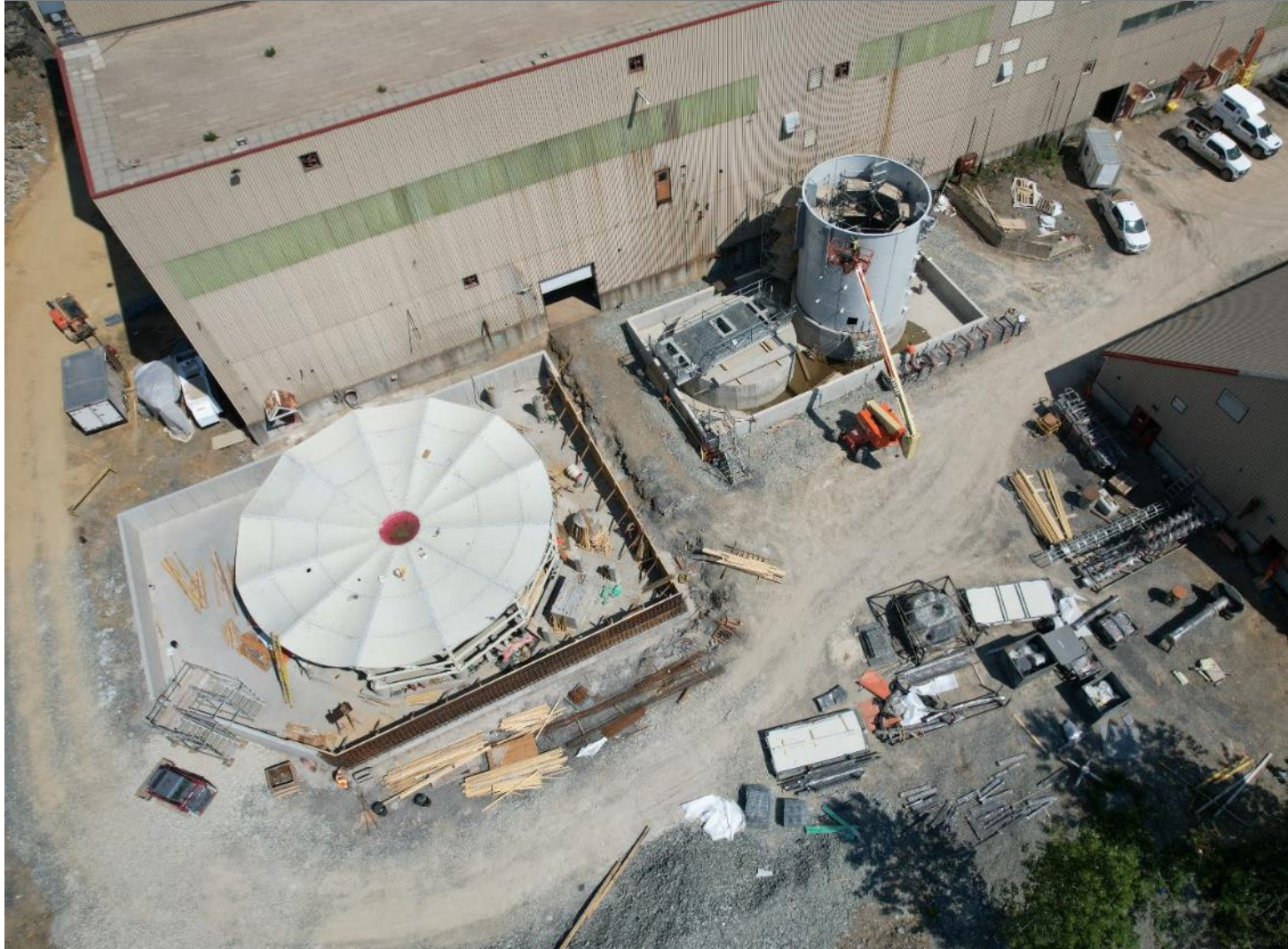
Tailings thickener and CN destruction tanks
