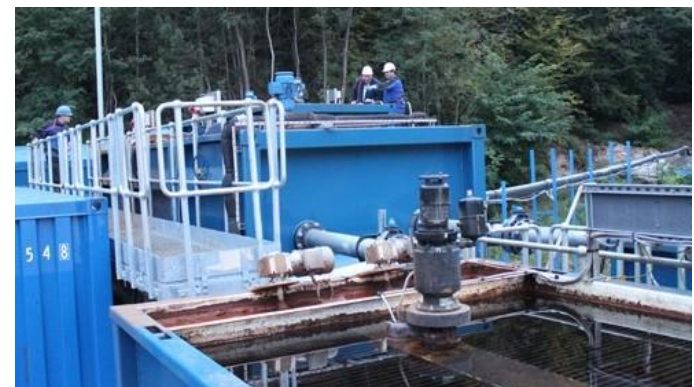
Water treatment facility, fully operational
