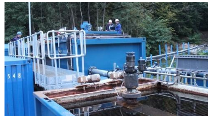
Water treatment facility, fully operational
