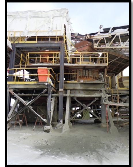
Secondary and tertiary cone crushers and screen plant at the QR Mill Facility
