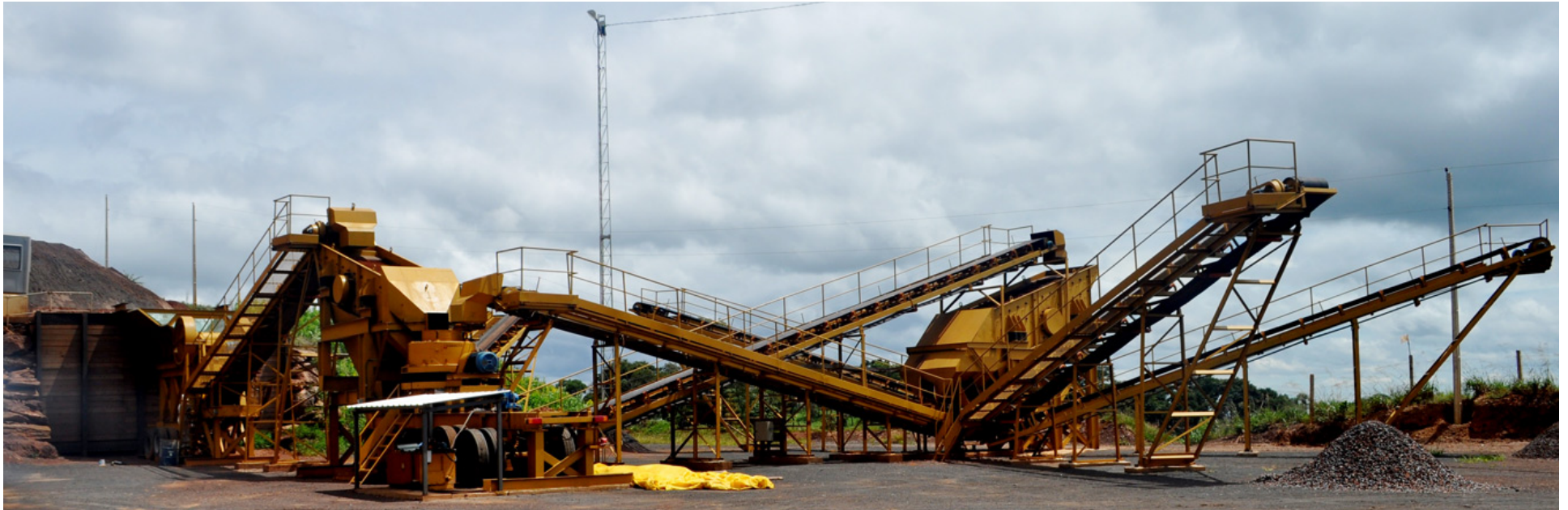
Posse plant fully commissioned and ready to start treating ore
