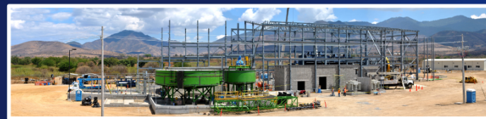
1,500 tpd Processing Plant
